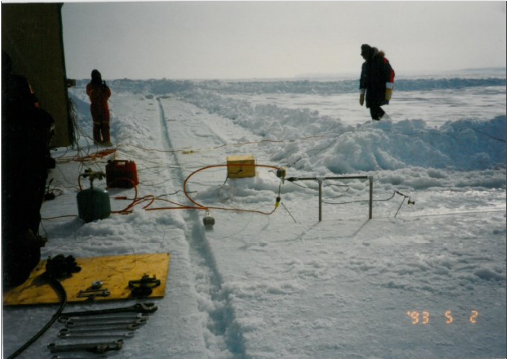
Pipes of a hydraulic flat jack inserted into a 24 m narrow notch, emanating from one edge of 80 m x 80 m square specimen, whose one edge is visible. The jack is driven by computers located in the cabin at left.
